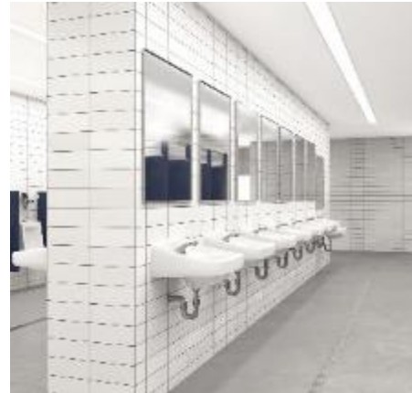
Touch-free Faucets & Soap Dispensers Toilets and Urinals
